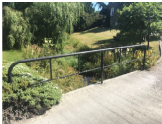
View of existing concrete bridge leading to Parochial House depicting the balustrade that poses a safety risk
