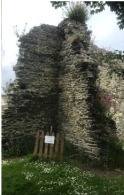
View of part of Abbey remains where projecting parts are vulnerable to damage and in need of protection from direct access, involving railed protection
